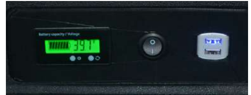
Battery Monitor, Light Switch & USB Port (no cover)
